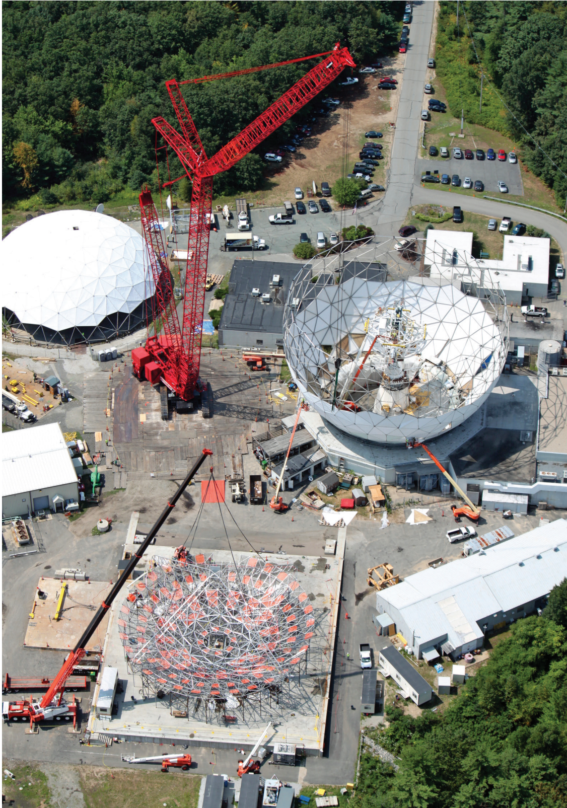
This aerial view shows the HUSIR construction site in August 2010 just before the installation of the new backstructure. The 400-foot-tall main crane towers over the truncated radome and the radome cap (upper left). In the foreground, a smaller crane lifts the quadrapod onto the backstructure.
