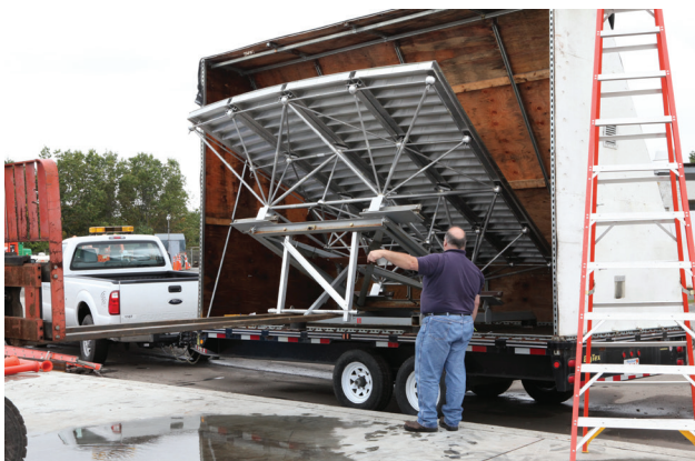
FIGURE 41. A subframe is secured to the steel frame on the transport trailer and then pivoted to fit inside the 8-foot-wide trailer body.
