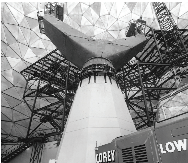
FIGURE 2. Mobile cranes and extensive scaffolding were used to build the original Haystack antenna within the confines of the radome.
