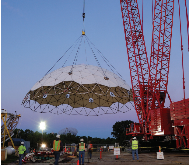
FIGURE 14. The cap was lifted off the Haystack radome and carefully swung to its temporary landing site.
