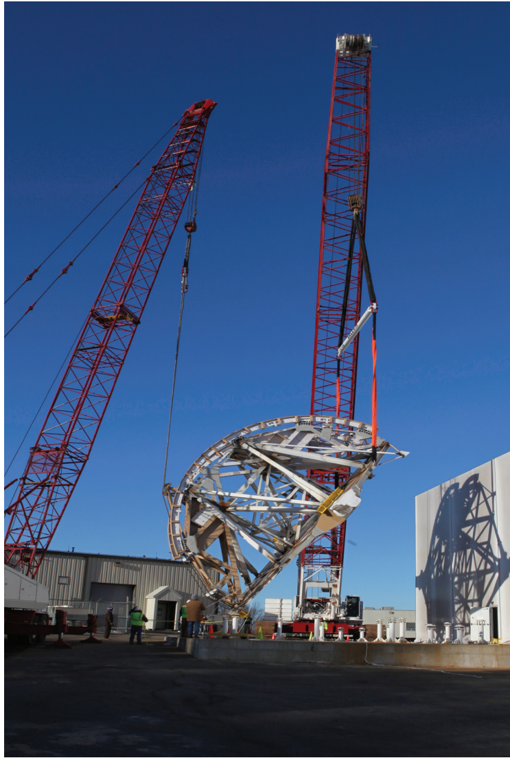
FIGURE 23. During a tandem lift operation, the transition structure is inverted and moved from its face-down assembly area to a pair of supporting tripods where final integration continues face up.
