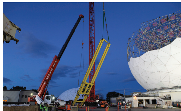
FIGURE 33. The rails and dolly for the RF box insertion system are raised up in preparation to be threaded down into the transition structure.
