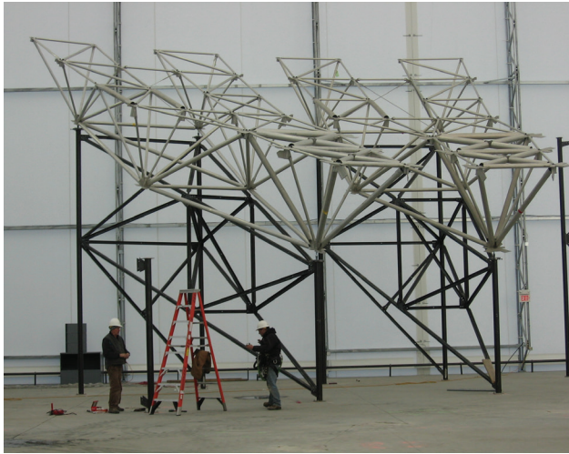
FIGURE 26. The first two radial rib sections are installed on their assembly stands inside the temporary building. Note the workers and the 8-foot stepladder for scale.
