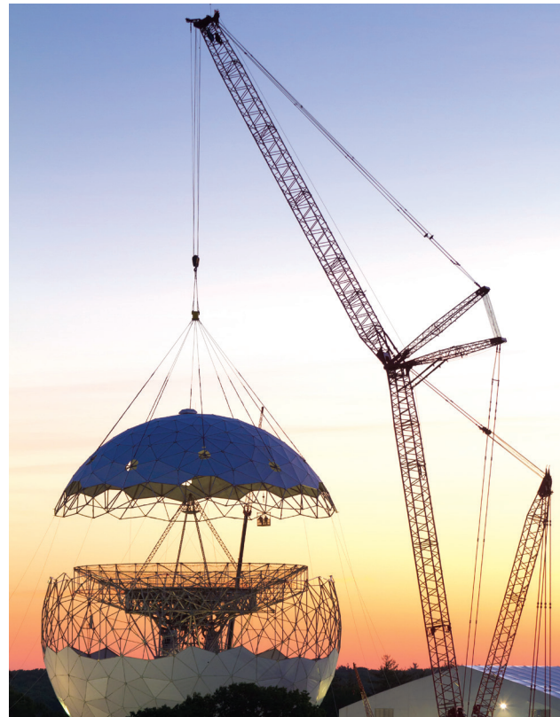
FIGURE 13. The 400-foot-tall main crane and smaller support cranes are silhouetted against the sunrise just after the radome cap is lifted. Photograph by Colin Lonsdale.
