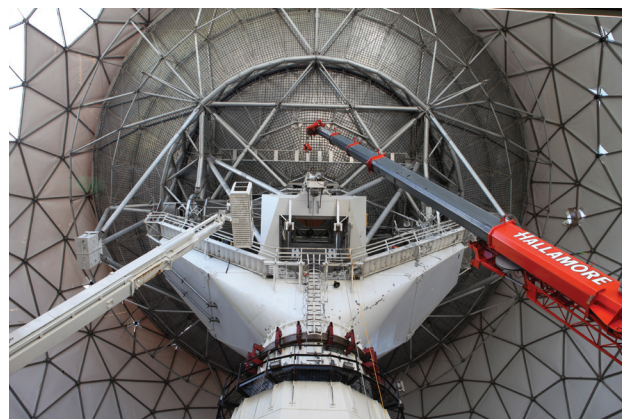
FIGURE 6. A crane connected to the 30-ton counterweight compensates for the missing RF box as the antenna is rotated to zenith for the last time.
