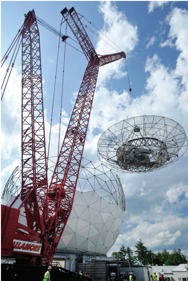
FIGURE 15. The 43-ton old backstructure was lifted over the edge of the radome and set down behind the temporary building to await demolition.
