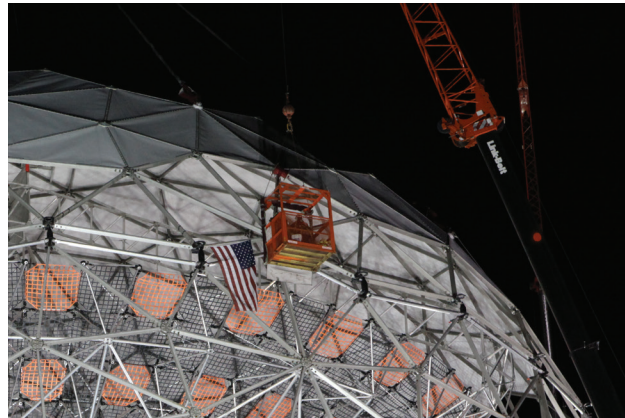
FIGURE 36. Workers in aerial lifts and crane baskets guide the radome cap onto the truncated radome.
