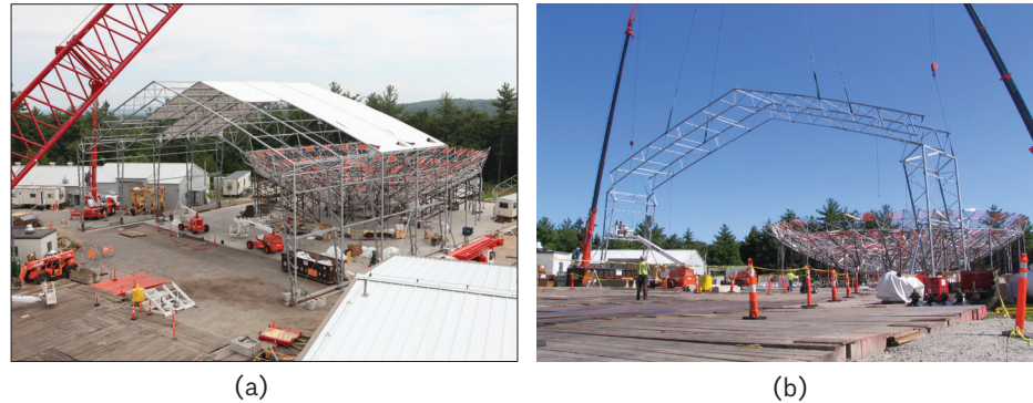
FIGURE 31. (a) Removal of the temporary building involved setting the building on rollers and rolling it into the parking lot for removal to minimize risk to the newly built backstructure seen in the background in (b).
