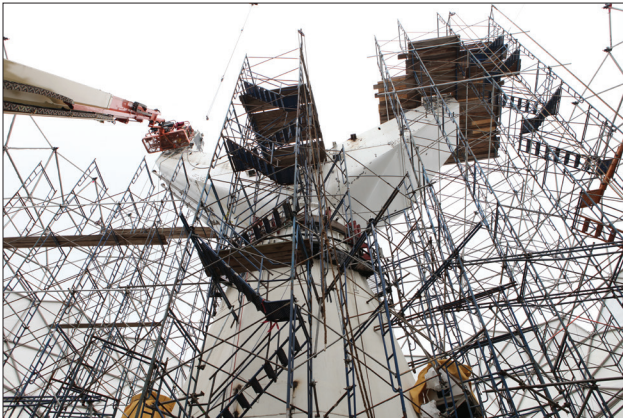
FIGURE 19. Towers of scaffolding ascend from the floor of the radome as the yoke structure is stripped of old components and modified to accept the new transition structure.
