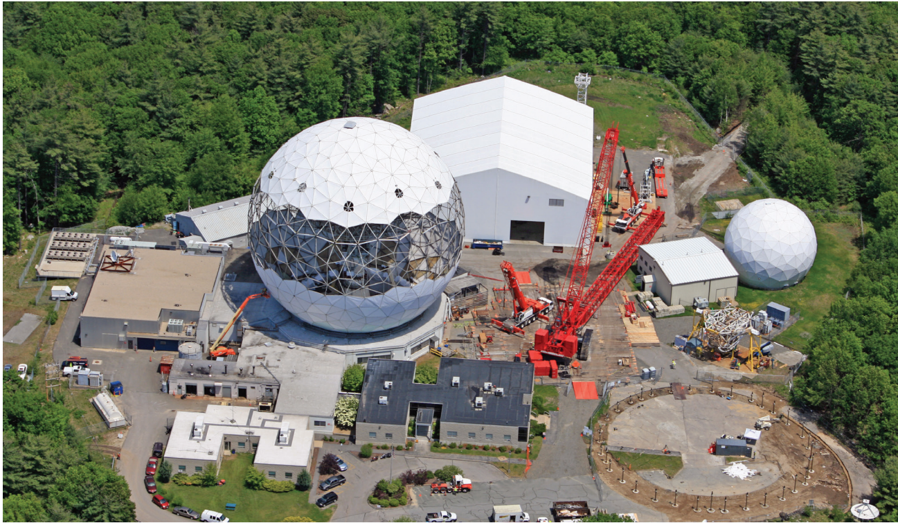
FIGURE 11. The assembly of the heavy-lift crane takes place along a 400 ft roadbed built into the treeline while the radome membranes around the equator are removed in preparation for the separation of the radome cap. The temporary landing zone for the cap is the ring of steel piers in the lower right corner.
