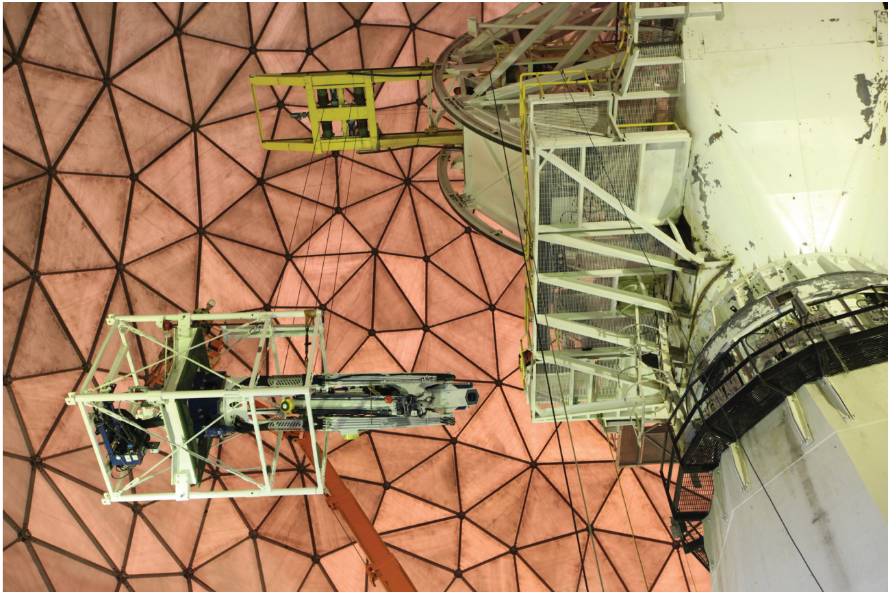
FIGURE 46. The RF box insertion system (RFBIS) hoist lowers the folded-up knuckle-boom crane down to the floor after completion of the subframe installation.
